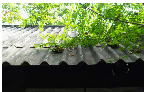
✗ Overgrown trees can cause roof damage.
