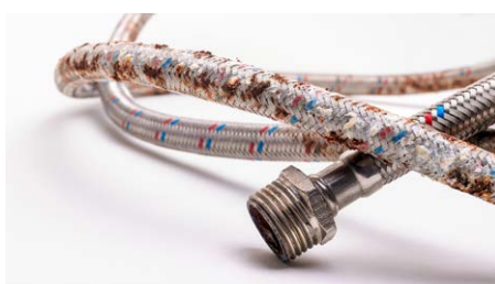
✗ Flexi hose in poor condition.
